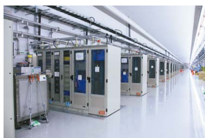
Fig. 2. Oil tank of the compact C-band oil-field modulator (left middle) and the racks to contain LLRF and timing systems in the klystron gallery.
