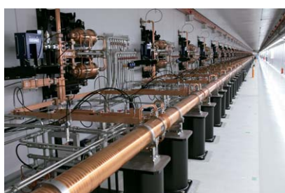
Fig. 1. C-band acceleration units installed in the accelerator building.
